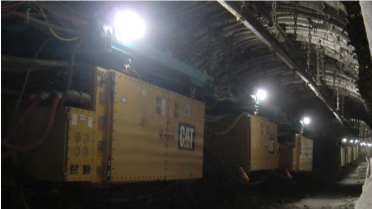
Figure 21. VFDs of the “Bogdanka” 2 plow system placed in the energy train on tail drive
