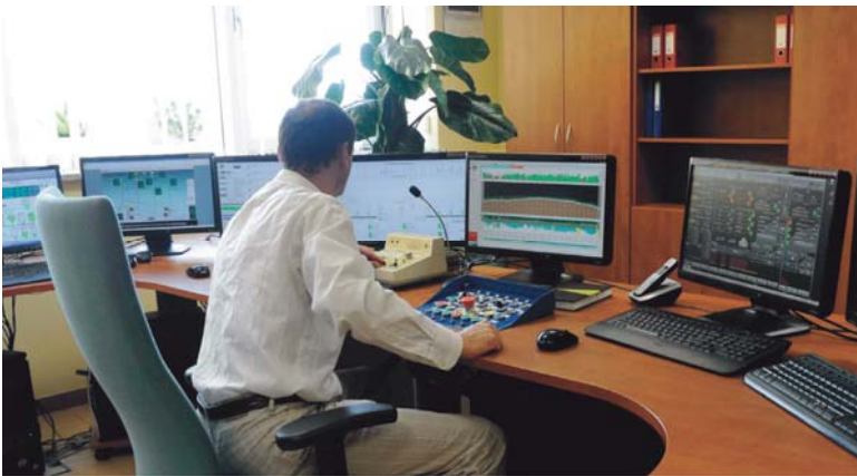
Figure 18. Plow control room on Stefanów
